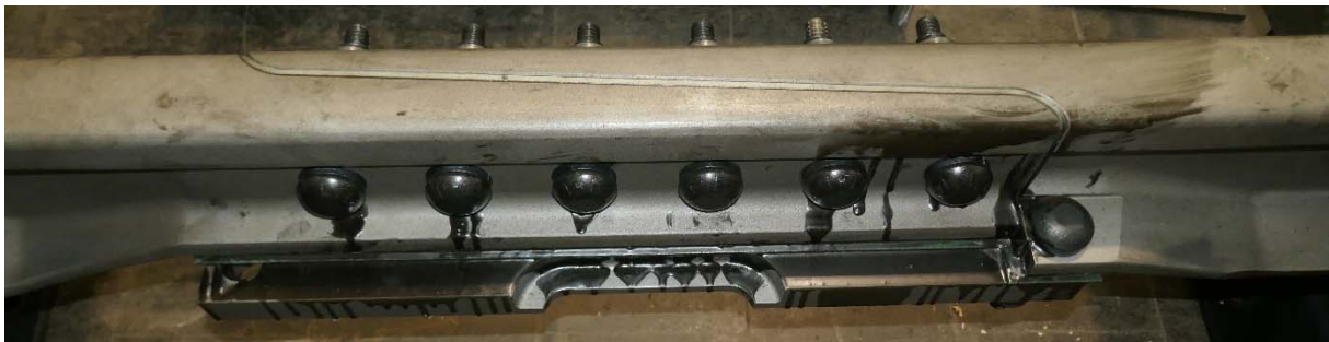
Figure 2: Opposite view of insulated joint "ABJ"
